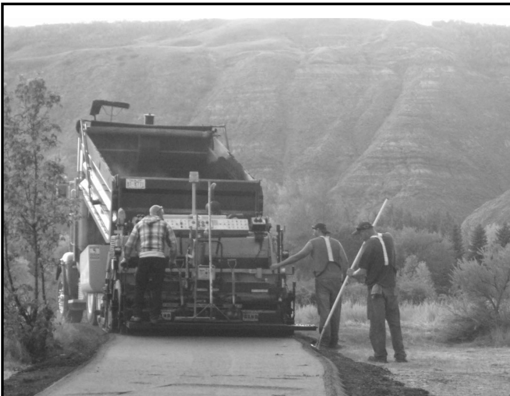
Town of Drumheller Project - Laying down asphalt on the trail connecting the town of Drumheller with the Royal Tyrrell Museum
