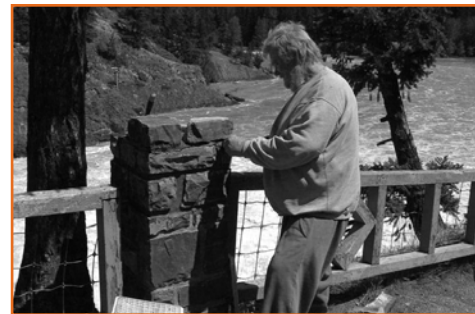
Stone Mason Herb Haupt, works to raise the height of the heritage stone posts to accommodate the new higher railings.
